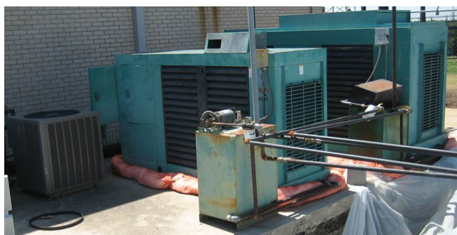
Existing emergency generation equipment at the Oncor facility's site.
